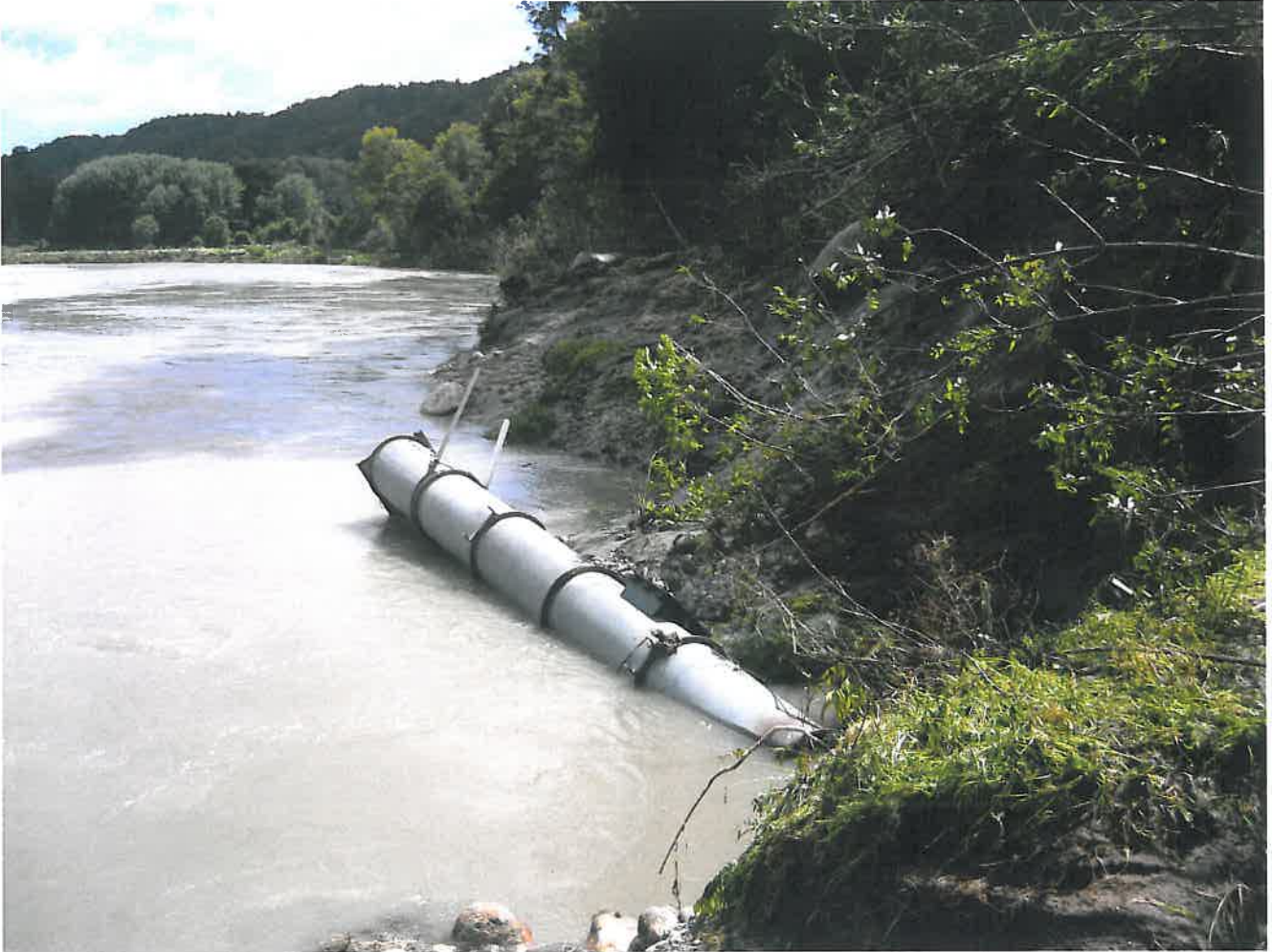
Figure 1: Tower from Ahaura River at Gorge. The tower will not be replaced, instead a gas bubbler system will be installed when the flows are lower this summer.
